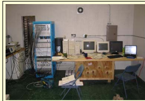
Inside the Control Shelter
